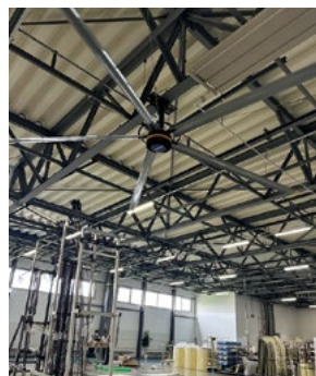
Preventing heatstroke at the Gotemba Plant: Large, energy-saving fans
